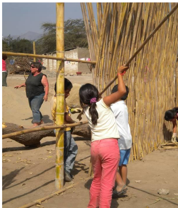
FIG 10: Children learn to build a cane fence using a common local technique
